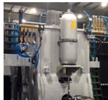
The machine was connected to several monitoring devices during the trials.
