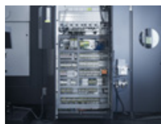
Climatized electric cabinet with easy access.
